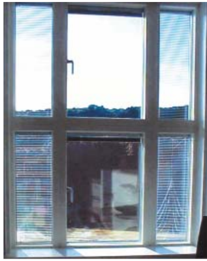
Figure 9 Breakage of inner glass in units with Venetian blinds
